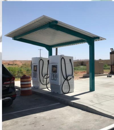
EV Charging station located at the AM/PM in Glendale, NV
